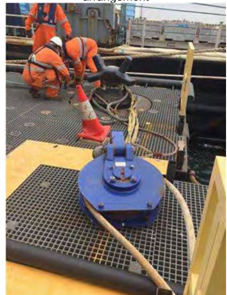
Sheave block came to rest on Walkway
