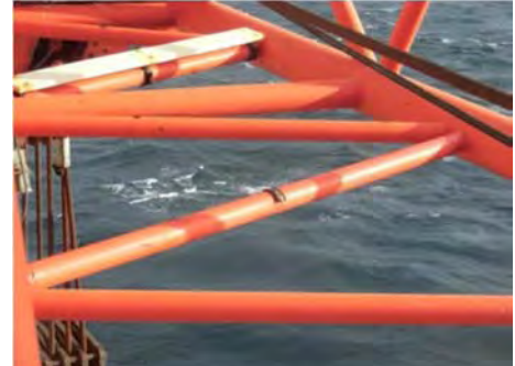
Original position of Teflon wear plate on boom lacing in boom tip section
