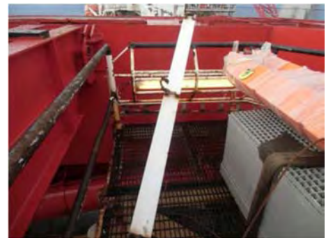
Fallen wear plate on C Deck adjacent to the load landing area.
