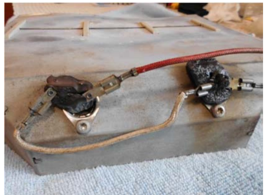
Damage to safety cutouts
