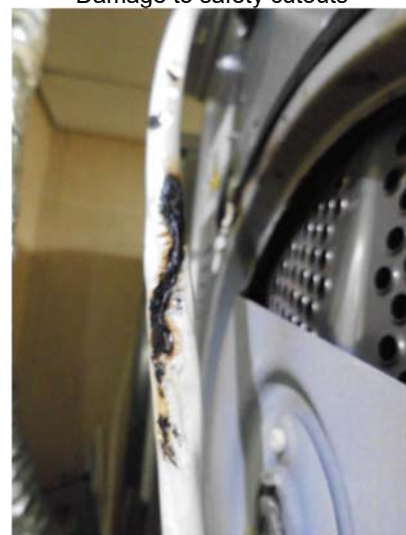
Damage to power lead
