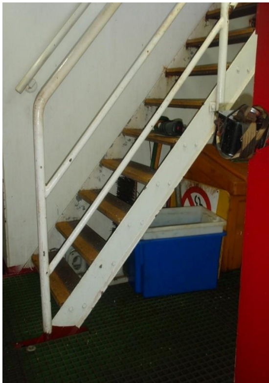
Photo 2 – Position of the hazards on the 5 th step tread from bottom.
